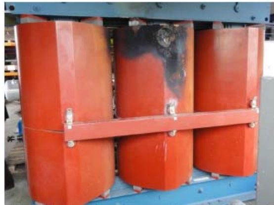
Fig. 8 Dry-type transformer with winding to leads fault on the middle phase
